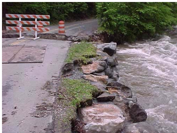
Tremont Road undercut and washed out.
